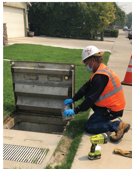
A worker from the Consolidated Mosquito Abatement District in Fresno County treats a utility vault to eliminate breeding areas.
